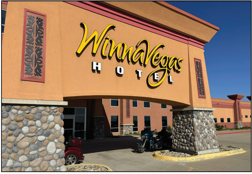
A complete refresh for the exterior of the hotel tower was completed. This was the first major maintenance project since the hotel opened in 2012! Followed by the entire hotel exterior painted and restored to its original colors. Work expertly completed by Ho-Chunk Construction, under the direction of Mr. Jamie Chamberlin from HCI.
