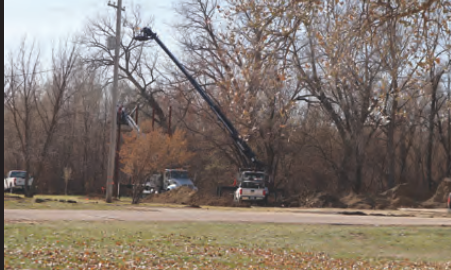
A lot construction is currently taking place in Winnebago! Here is an updated look at the installation site for the big screen projector that was put in place for streaming COVID response videos, Tribal Council meetings, and other live streamed updates.
