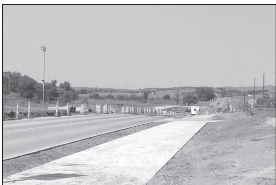
Here is an updated look at the progress with construction that is taking place on the main street through Winnebago, Bluff St.
