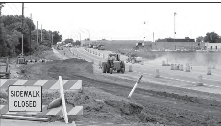
North of Winnebago construction zone is now alternating traffic with the use of stoplights and expanding for more work to be done near the 2nd roundabout worksite.
