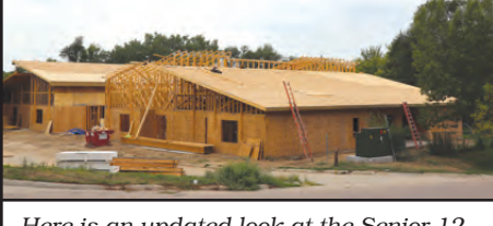
Here is an updated look at the Senior 12 plex project and the progress being made. You will find more construction updates in this issue!
