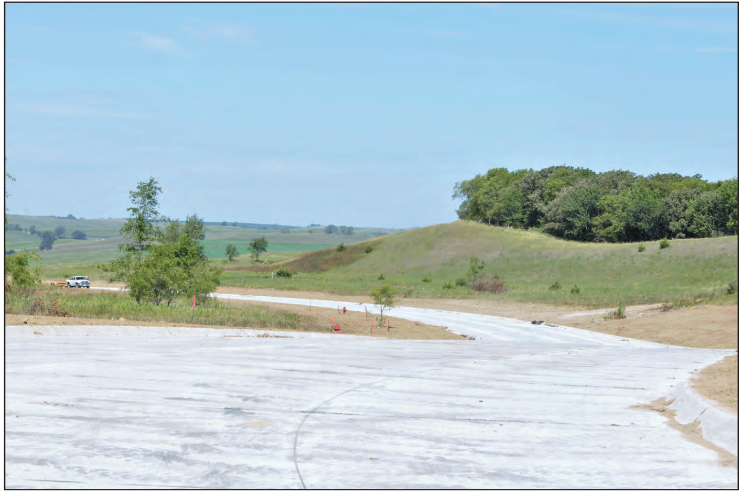
The quarantine housing project is the biggest project funded by the CARES Act money. Here is a glance from the top of Big Winnebago Lane at Thunderway where the housing units are being built.
