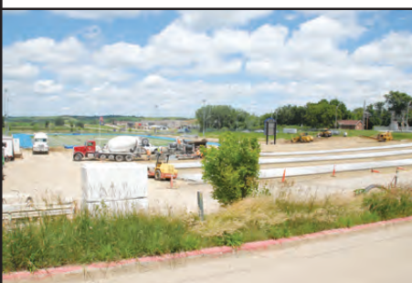
Concrete was flowing of out trucks this past week for WPS's new larger parking lot.
