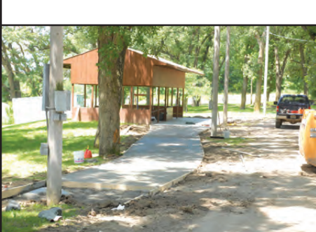
More concrete was being poured out at the Veteran's Memorial Park to connect the existing sidewalks. Now those kids can go round and round without dusty shoes.
