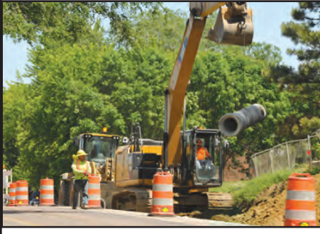
A hot summer day was not going to slow down these two workers, as they continued to work hard through the heat. Read more construction updates in this issue!
