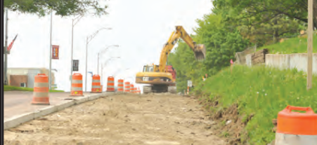
Construction throughout Winnebago is currently in progress! HWY 75/77 workers, right in front of WPS, has adjusted their work zone area to accommodate oncoming traffic. (Construction updates will be included in our next issue.)
