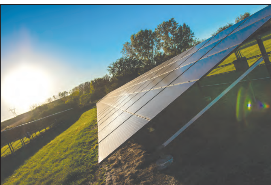
The Winnebago community's investment in renewable resources – including boasting more than 2,400 solar panels – has helped it save almost $250,000 in a little more than a decade.
