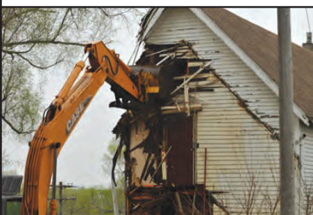
On May 4th, the old halfway house was demolished by our Tribal Roads Department. The building was over 100 years old; construction on a new halfway house will begin soon.
