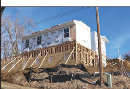
One of the current ongoing construction projects in Winnebago is the new Halfway House; here is an updated look at the progress being made.
