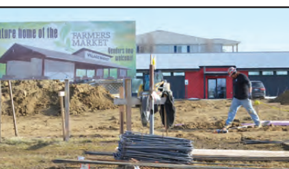
Construction has begun on the New Farmers Market building in the HoChunk Village. Area crafters and during the growing season will have a place to sell their personally grown farm produce.
