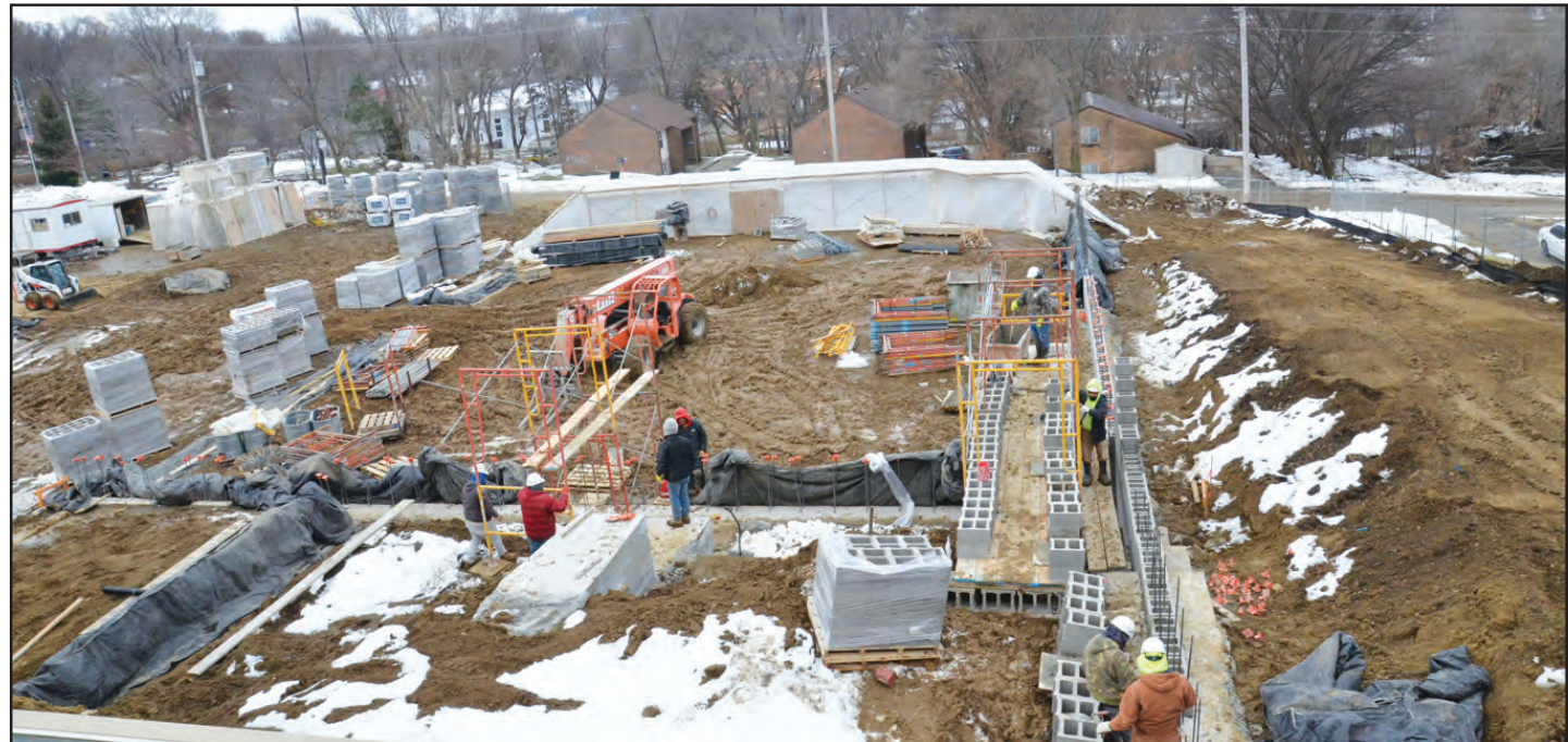
An updated look at the new classrooms currently being built on the south side of the Winnebago Public Schools. Work continues during the cold weather.
