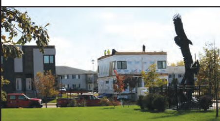
More housing Development is going up in the first stage of the HoChunk Village.
