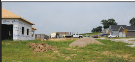
The Houses keep going up in the Ho-Chunk Village, here two new houses are going up east of the statue garden.
