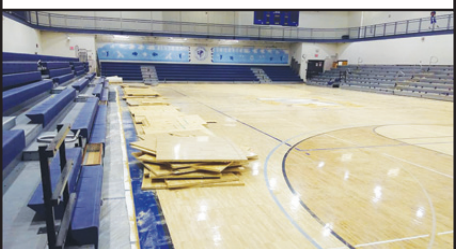
The WHS gym is being demolished this summer for a brand new floor coming in the Fall.
